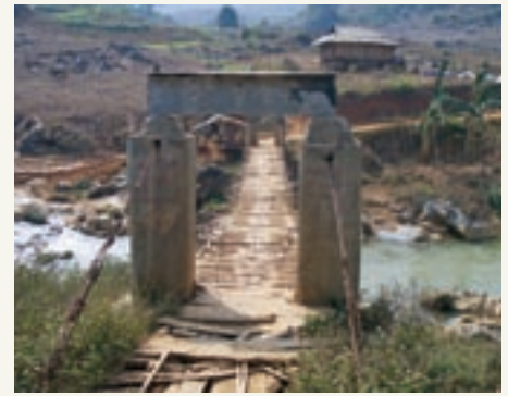
One of many bamboo suspension (and swinging) bridges the project team had to cross to visit remote village primary-school classrooms that will be rehabilitated by a project involving the Canadian International Development Agency, United Kingdom, Norway, Australia, and the World Bank.
